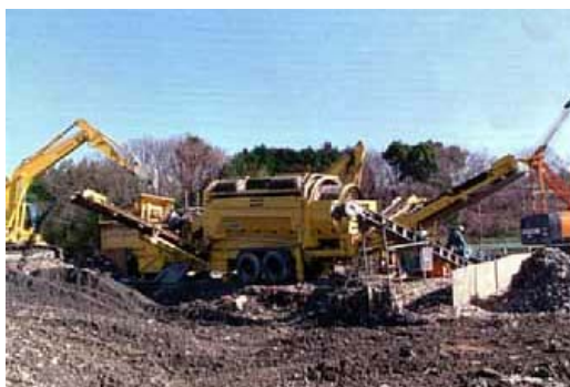
Mobile Waste Segregation Equipment
